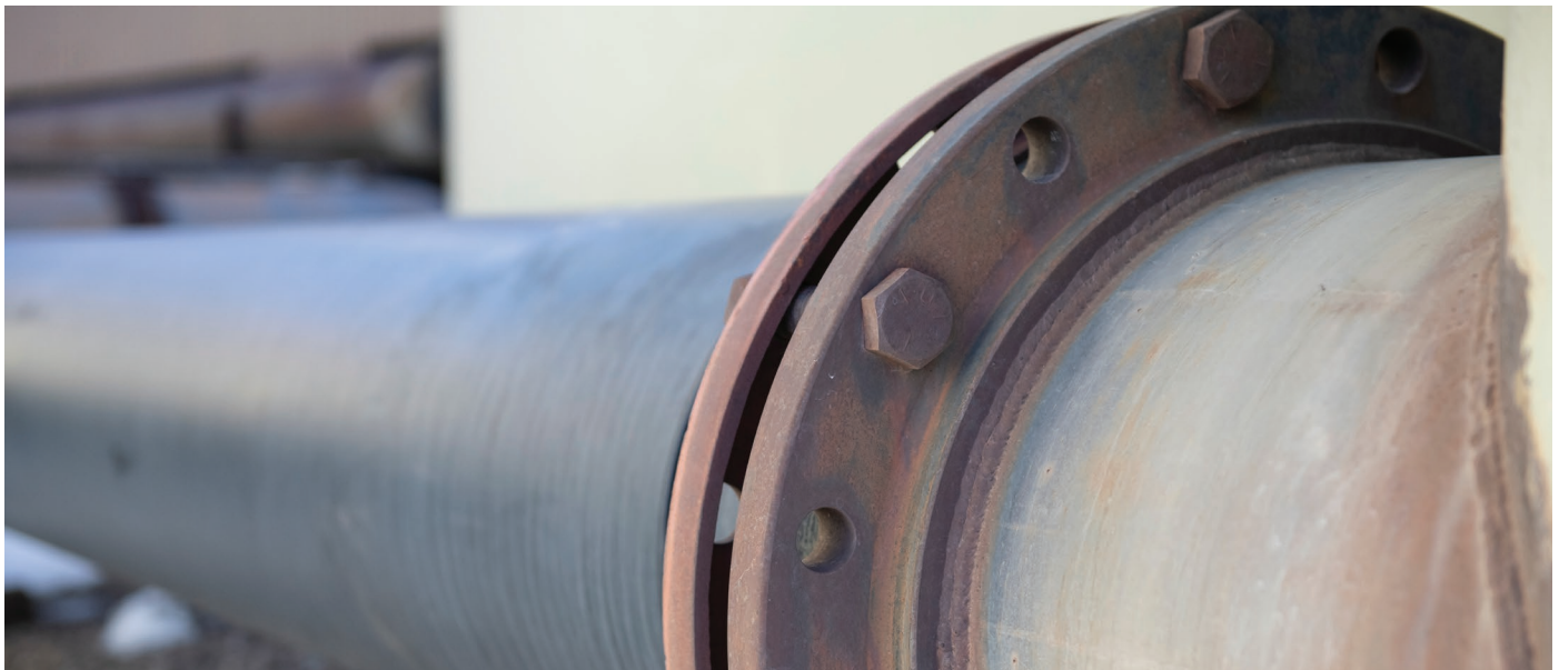
Large industrial horizontal water pipe
