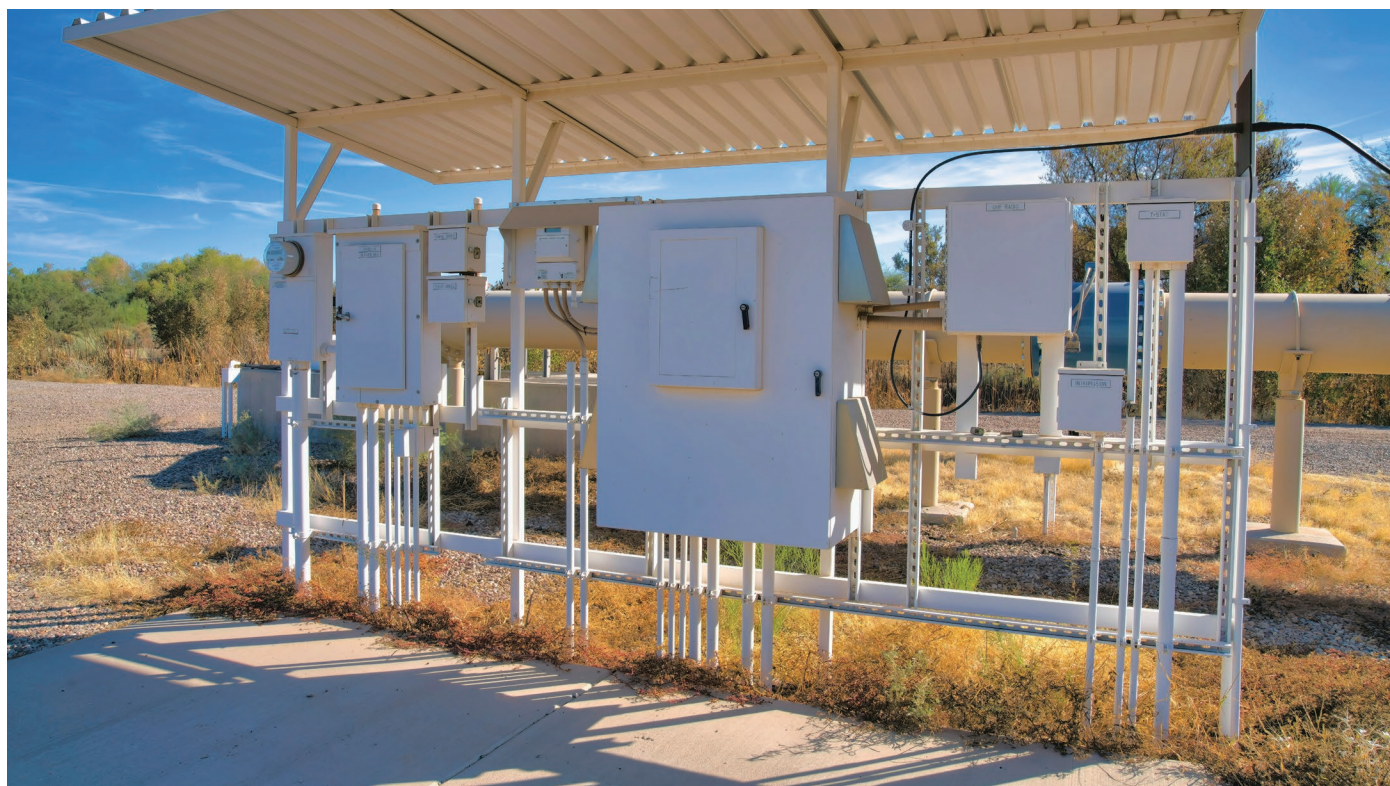
Sweetwater Wetlands electric water treatment utility infrastructure in Tucson
